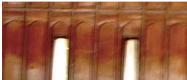
Plate 17. The semi-circular blind arches and ventilations of clear glass on the lower part of the west wall of the sanctuary.
