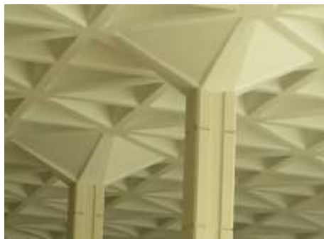
Figure 6. Coffered Ceiling and Capitals of the square piers in the ablution area.
