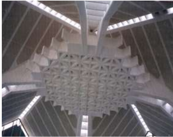
Figure 8. Perforated ceiling design set at the joining point of the girders and beams.
