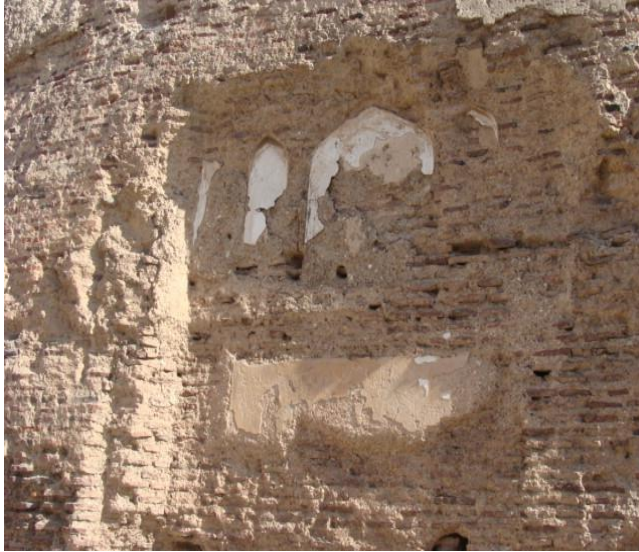
6. Wall, dressing room Shahjahani Hammam,Lahore Fort
